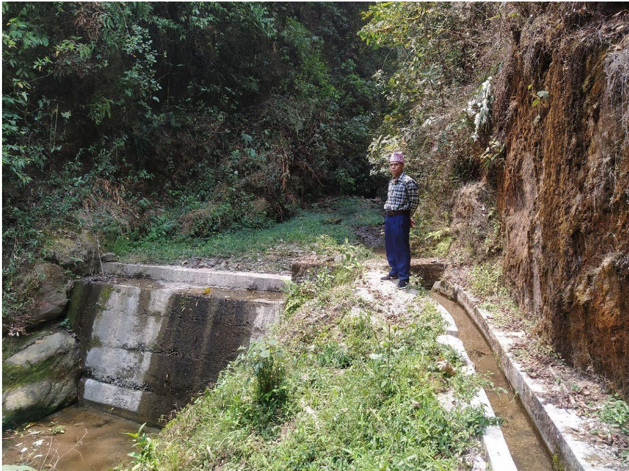
Annex Photo 13: Intake of Saanimai Kharibote Sana Sinchai IS in Ilam.
