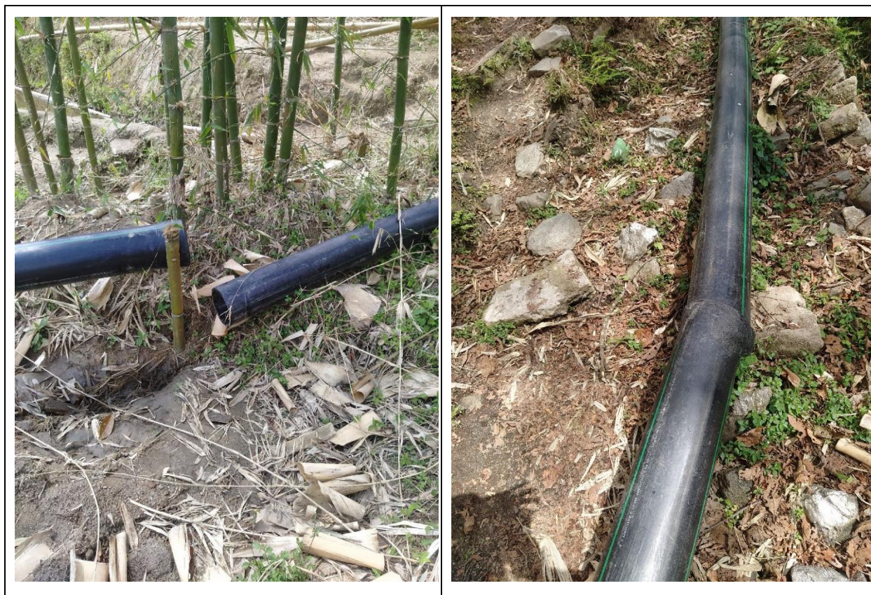
Photo 3-1: Examples of weak pipe joint a) Jaljale Chuchhe Dhuna Dobela IS, Khotang and b) Kharuwa khola Nali pipal danda rajkulo IS, Khotang.
