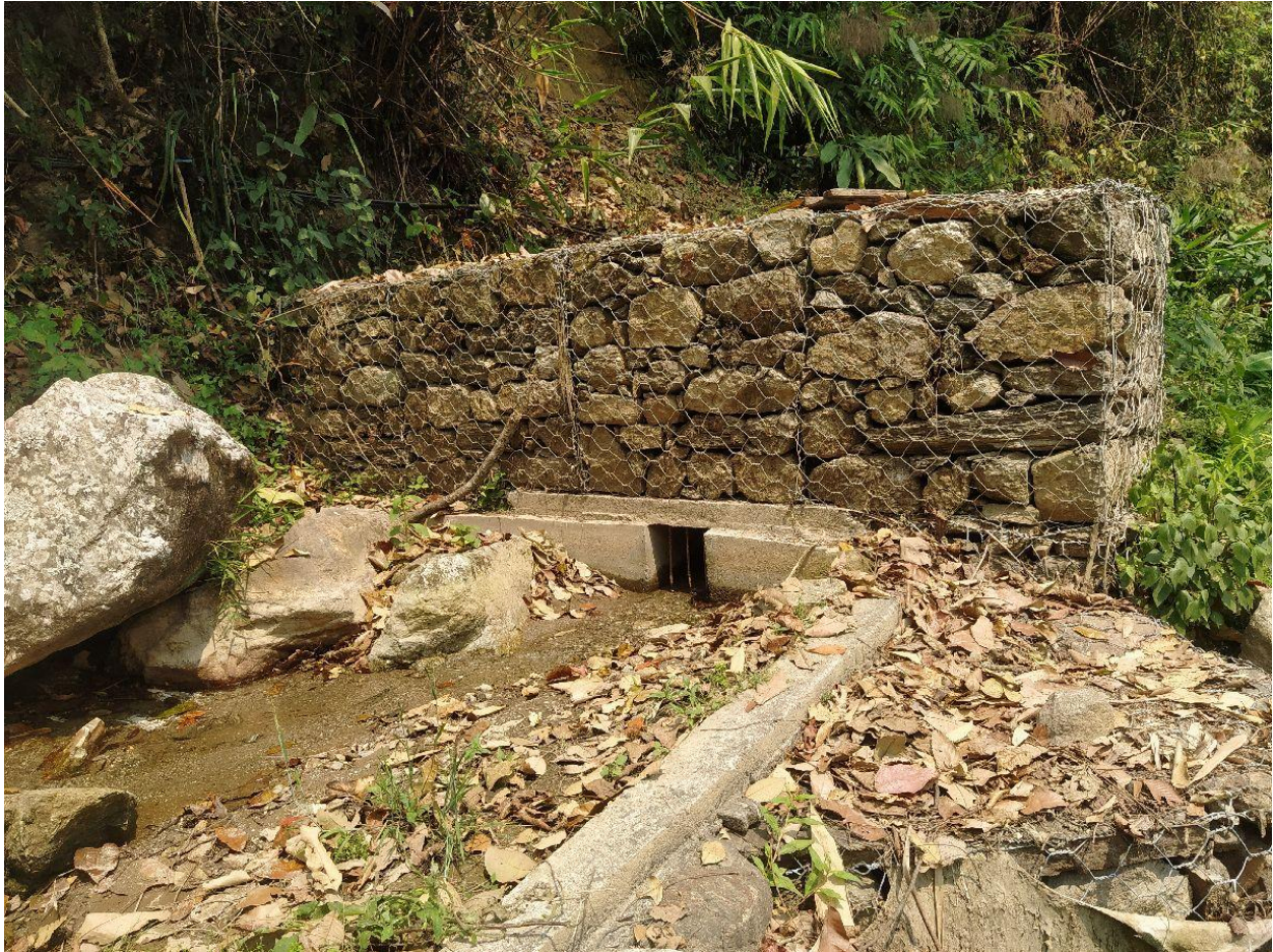
Annex Photo 14: Intake of Lewak Tole IS in Ilam District.
