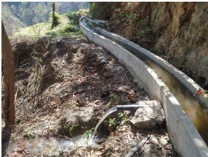
Photo 3-2: Release of water from outlet to slopes without proper protection in Khiku Khola Lamkulo IS, Khotang.
