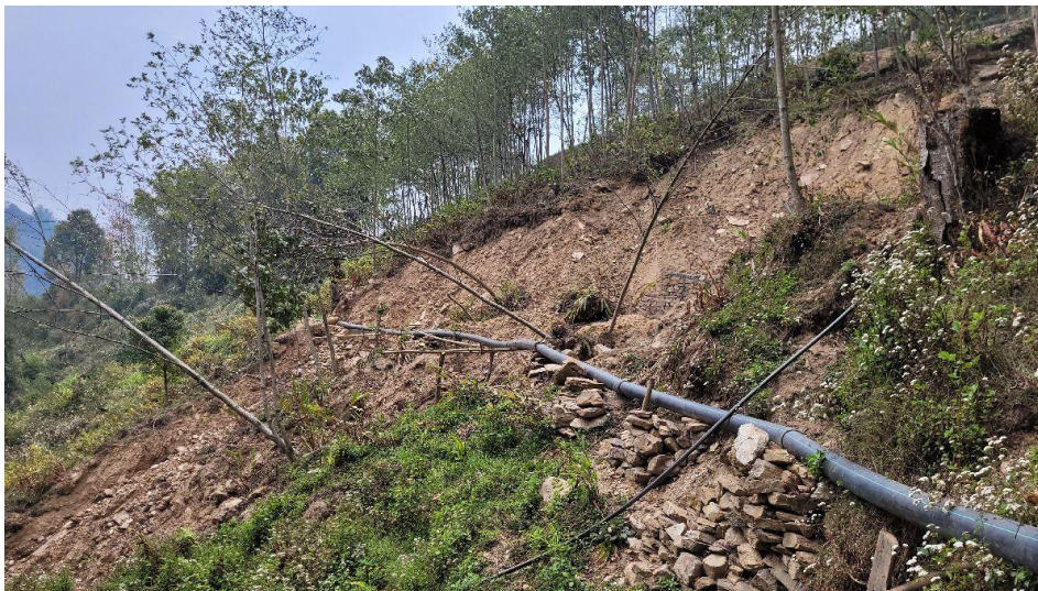
Photo 3-3: Pipe exposed to landslide and in vulnerable condition in Siran Kulo IS, Bhojpur.
